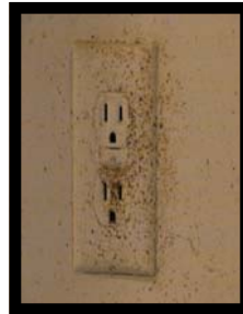
Roaches so bad they covered the outlet.
